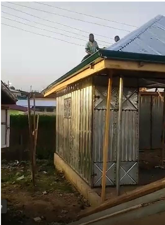
Picture 2: Side view, roofing of the milling centre at Amponsah Market, Suhum
