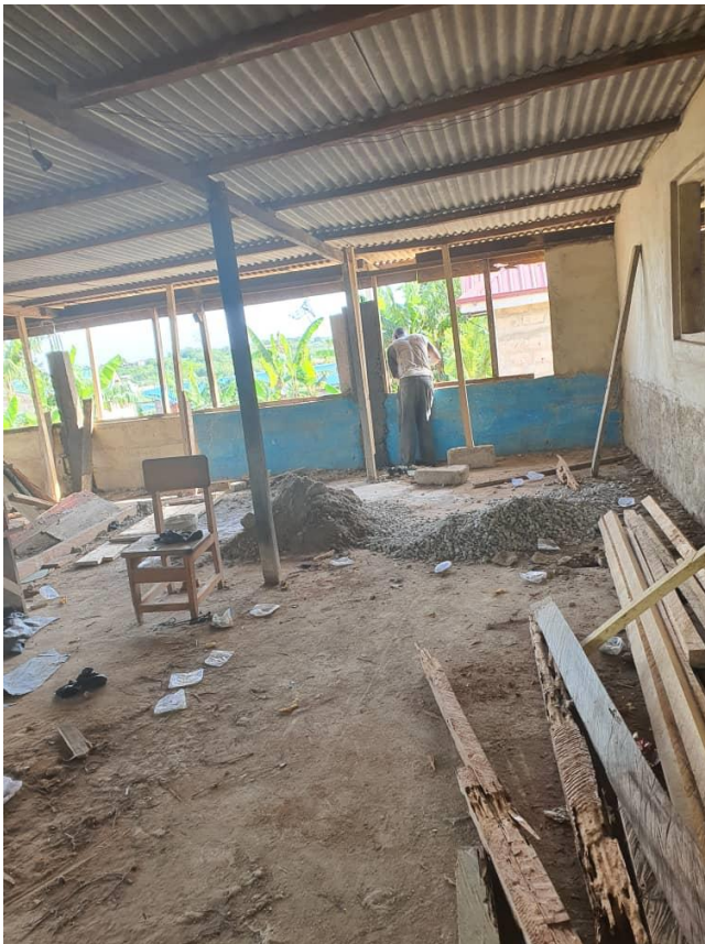
Picture 11: Reconstruction of the former school for people with hearing impairments for the water filling facility, Cape Coast.
