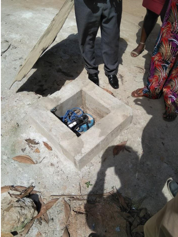
Figure 16: New 100 feet borehole to provide water for sachet water production, Cape Coast
