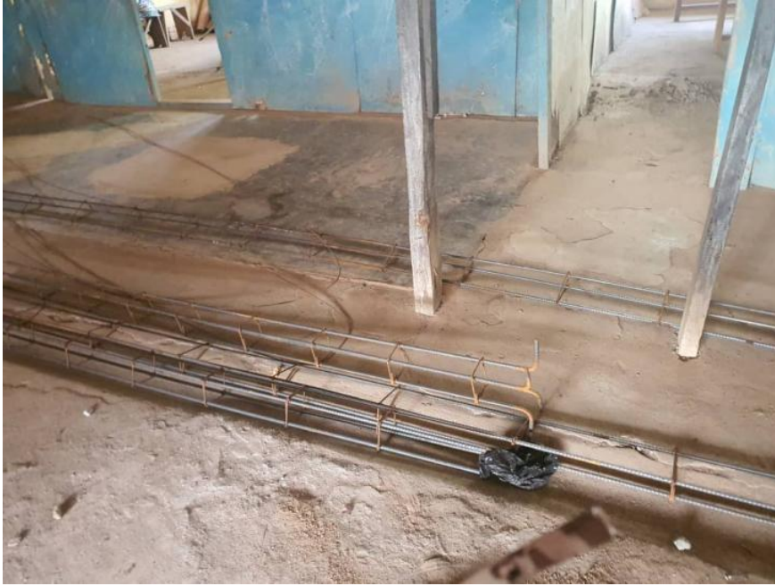
Picture 12: Reconstruction of the former school for the blind for the water filling facility, Cape Coast.
