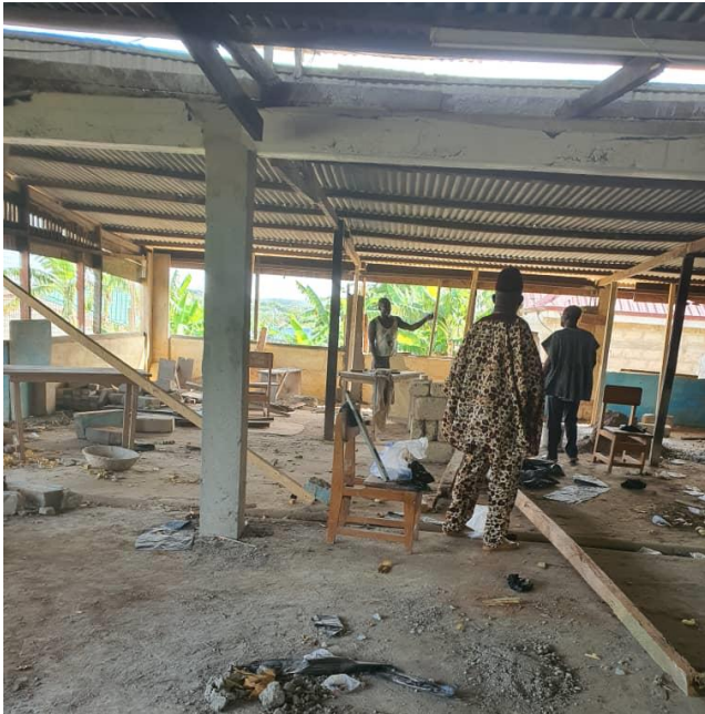
Picture 10: Reconstruction of the former school for people with hearing impairments for the water filling facility, Cape Coast.
